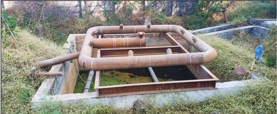
Rainwater Collection Tank installed at site
