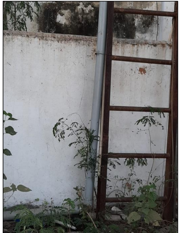
Rainwater Collection system installed at site
